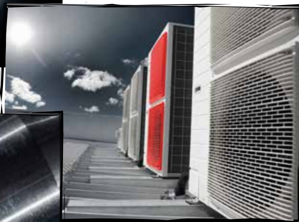
Heating, ventilation, air conditioning, and refrigeration (HVAC&R) applications
